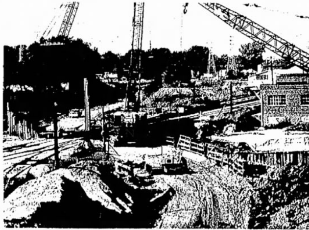
THE CUT-AND-COVER FLOOD PROTECTION conduit construction has reached the Missouri Pacific railroad bridge near Seventh and Main streets, Jerry Ashbach, Ashbach Construction Co., contractor on the U.S. Army Corps of Engineers project, said the entire project could be completed by the latter part of December.—Globe photo.
